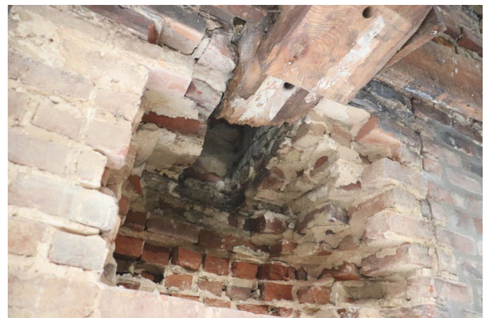
Figure 2: Deterioration of the wood trusses
